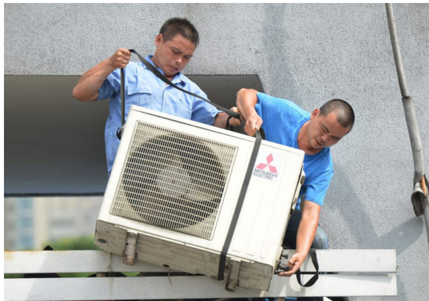
Workers install an air conditioner unit in a food store in Shanghai.
