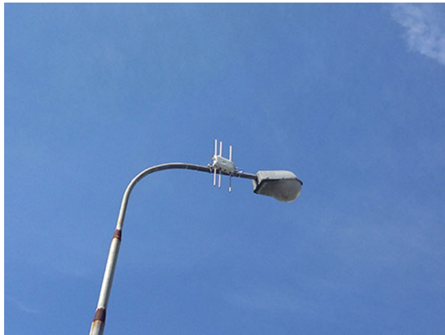
Photos of WiFi transceiver stations on the lampposts in Da Nang
