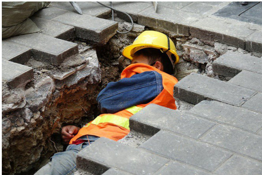
7. After hours of hard work, a construction worker took a nap in a roadside pit in Guizhou Province, China.
