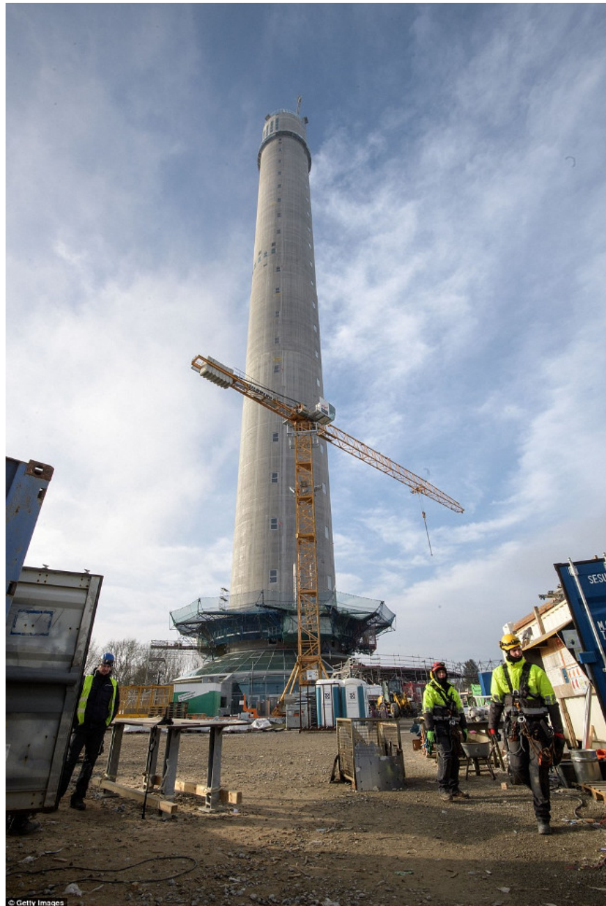
Workers are working under the newly built giant tower in Rottweil, southwestern Germany, where a new elevator system will be tested from next year .
