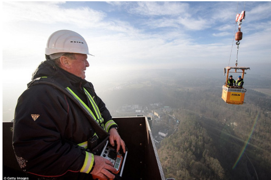
The crane operator - Peta Kustrta of Croatia is standing at a height of 236m and construction workers are bringing new elevators to test at the building.
