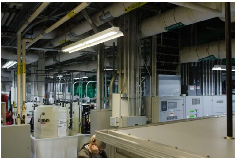
Titanium water cooling system.
