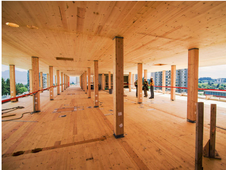
The interior of Brock Commons building is also made entirely of wood.
