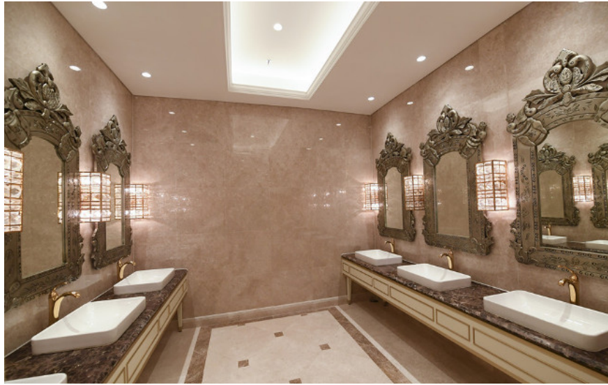
Toilet area next to banquet room with modern equipment, imported from countries with standards for 6-star hotels.
